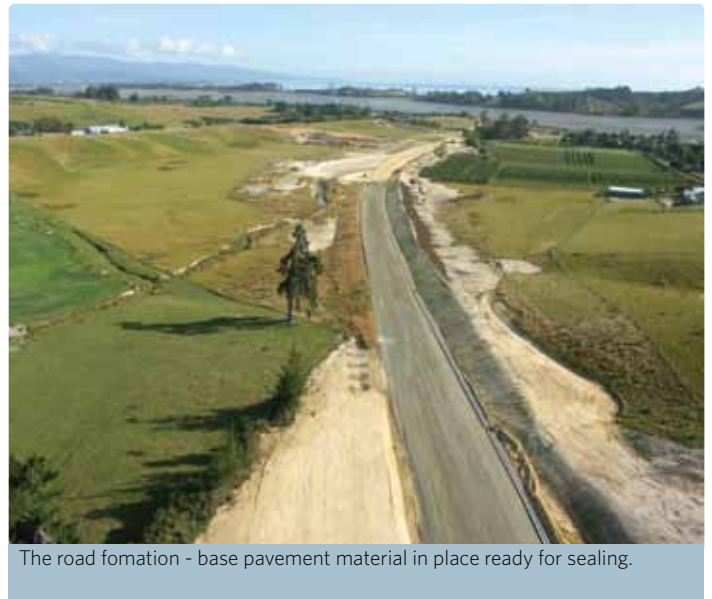
A temporary bypass has been created at Trafalgar Road to move traffic off the existing road.
