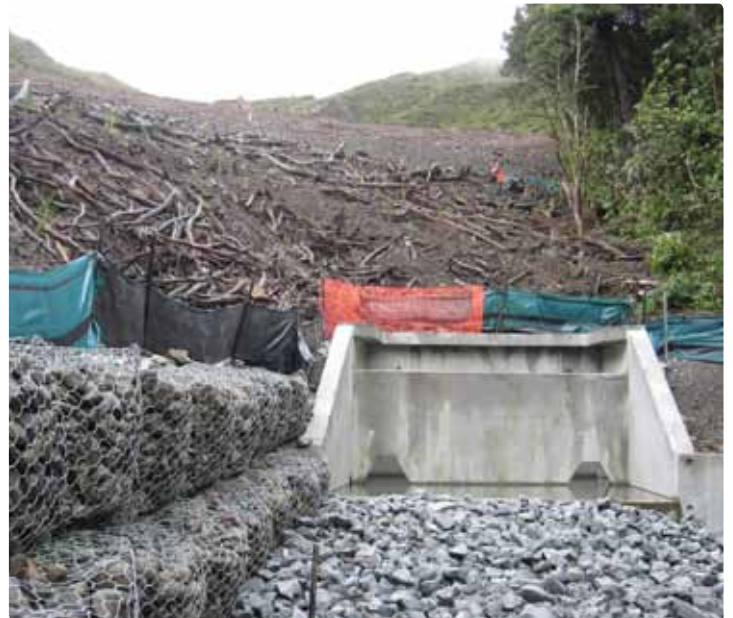
The stone-filled gabion baskets on the left help retain the fill slope as well as protect the stream at the bottom of the gully.
