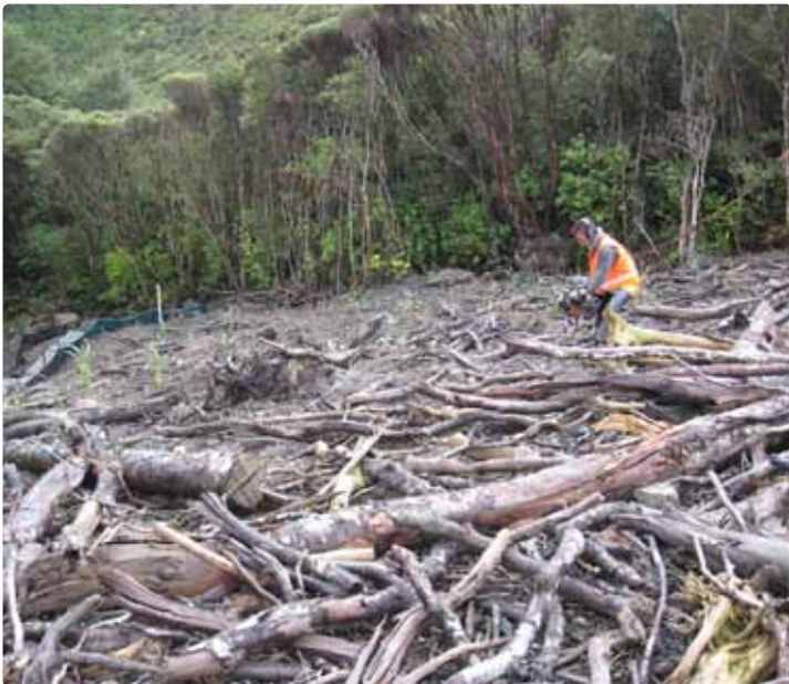
Forest debris is laid across the slope at fill site A and planting of natives such as flax has just began.
