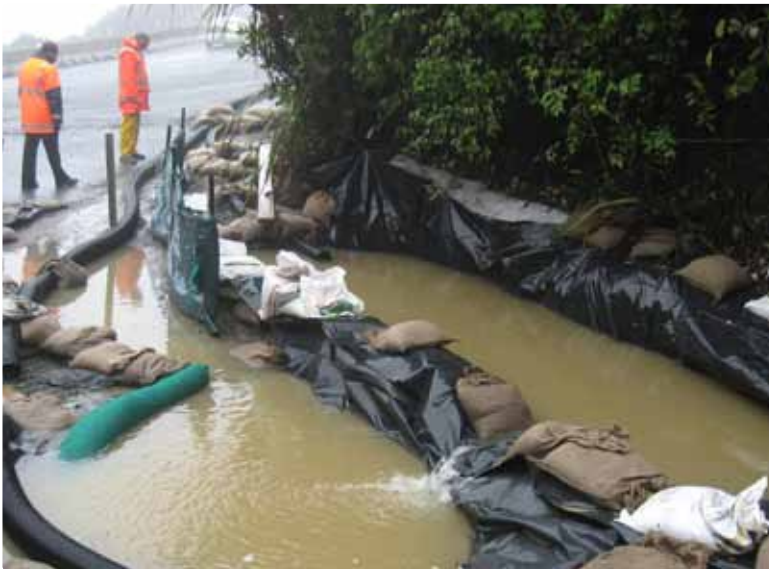
These are just some of the controls that help to keep sediment out of the streams and watercourses. The two holding ponds allow sediment to settle and clean water can then flow from the top of the ponds into the stormwater drains. Weather conditions have started to deteriorate but the NZTA project manager Simon Cribb (left) and Opus engineer to the contract Keith Atkinson made sure they were wrapped up against the elements when on site earlier this month.
