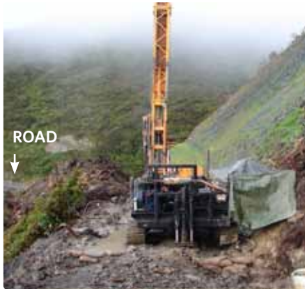
A borehole drill rig high up against the cut face of the hill monitors groundwater and helps to determine where rock anchors are placed in this area to stabilise the slope.
