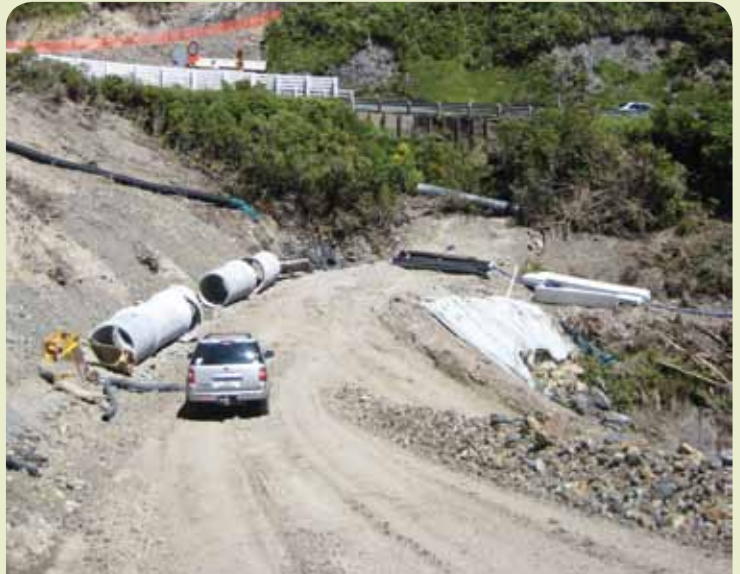
Sections of the 1.35m diameter pipe lined up ready to install as part of the new culvert which will be about 80m long and slope down a vertical drop of 25m.
